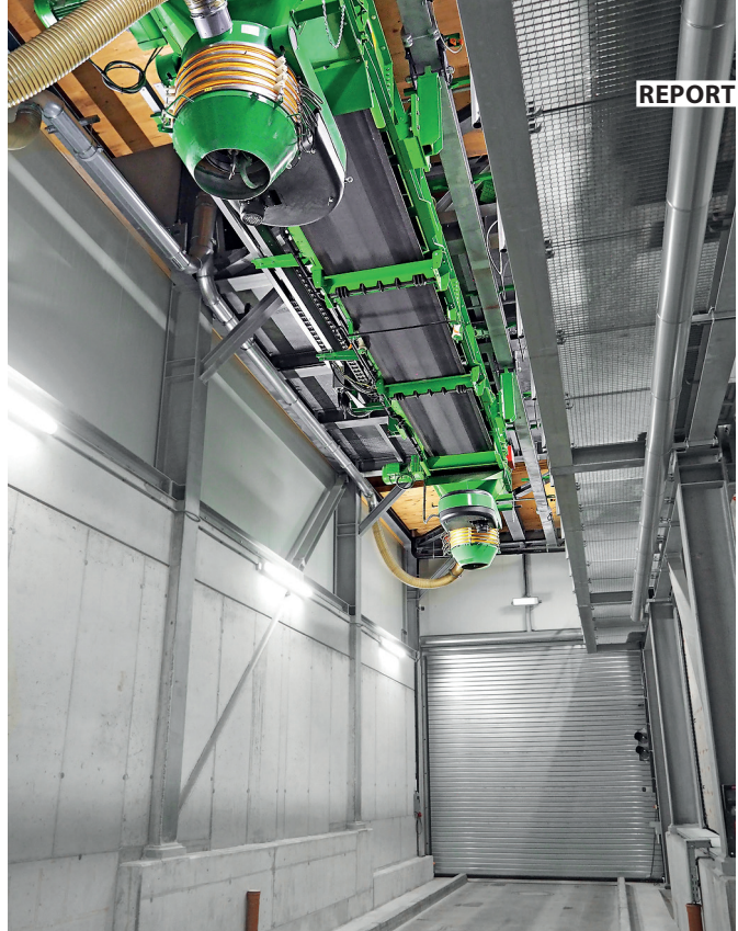
In order to meet the strict requirements for noise protection, a housing surrounds the entire loading station
